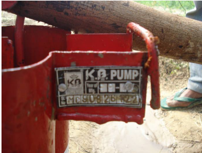
↑Punch Plate of Pump installed at District Baharich
