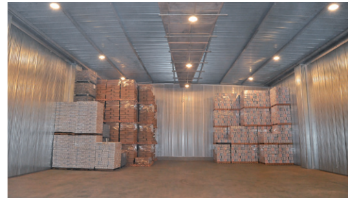
Post-repair, the Kesennuma freezer warehouse will eventually be able to store almost 170,000 tonnes of fish and seafood.
